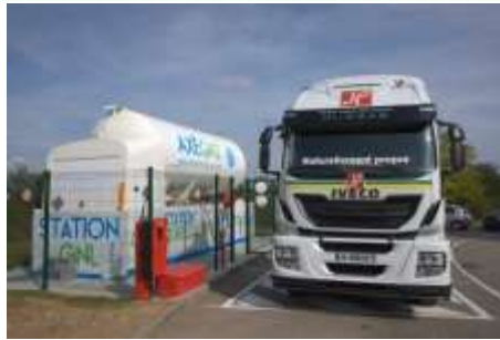
Station GNL de Saint Quentin Fallavier
